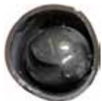
Damaged Check Valve
